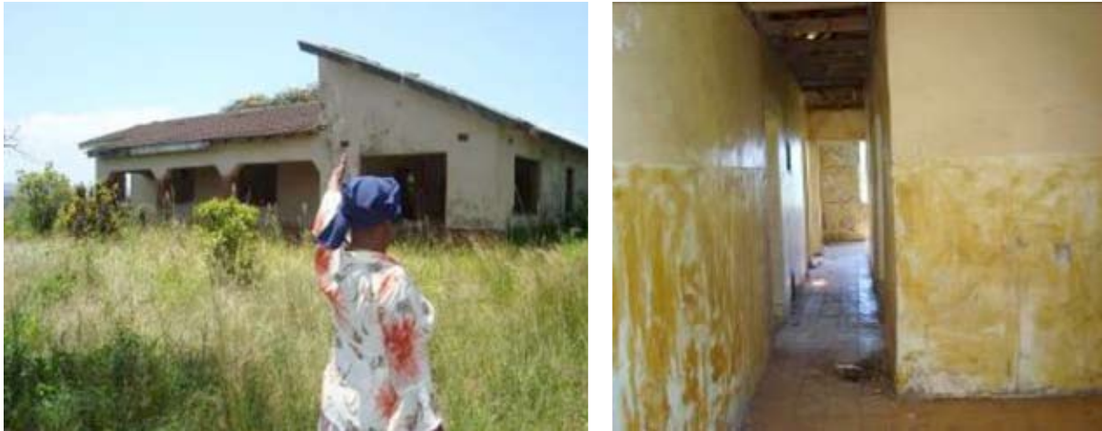
Figure 23: Failed Women's Project
